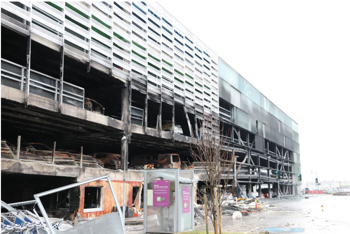
Figure 3-2 North-eastern part of car park after the fire. The left section shows building B and the right section building C.
